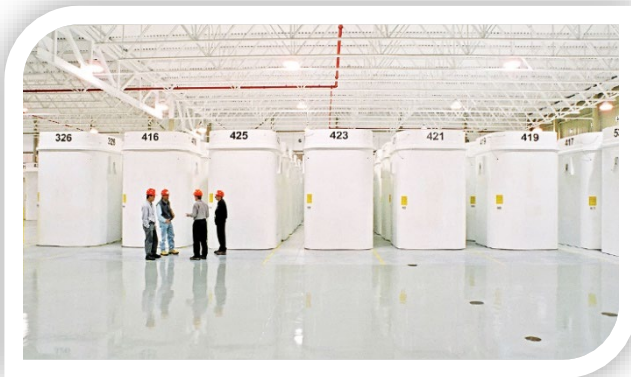
Dry Storage Containers are stored in simple warehouse facilities maintaining a suitable environment for long-term storage.
